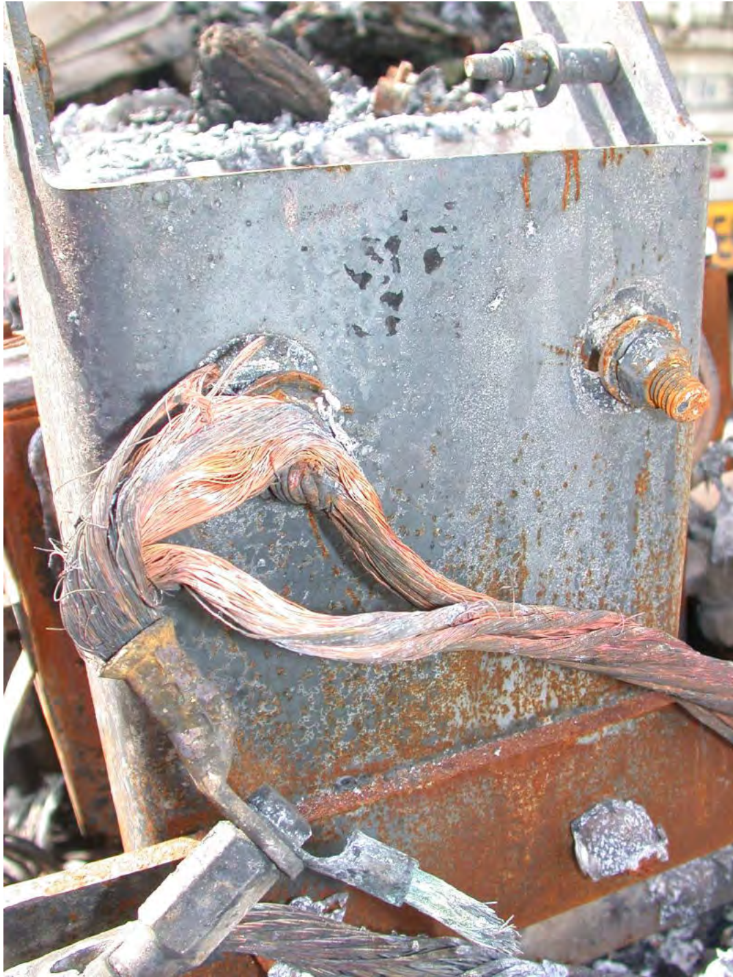
The result of a rub between a battery cable and the bolt that it was hooked over.
