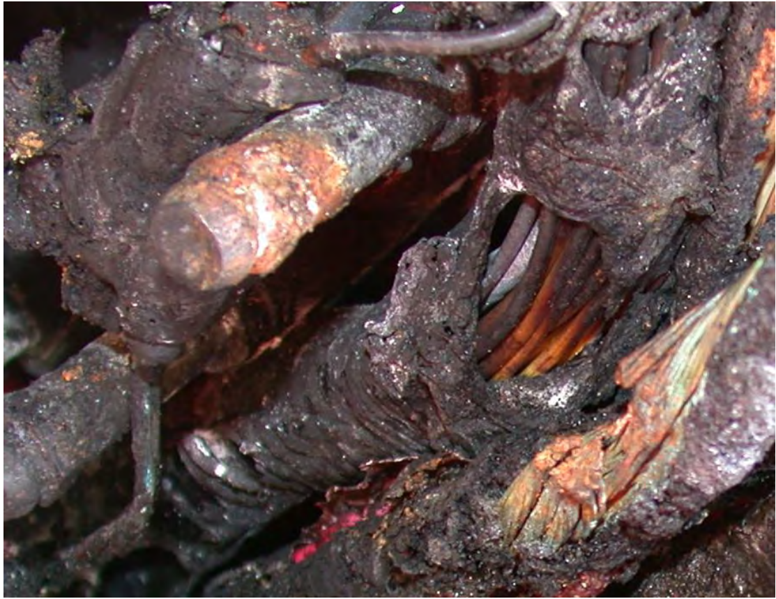
An engine compartment fire due to a rub between the alternator cable and the battery stud.
